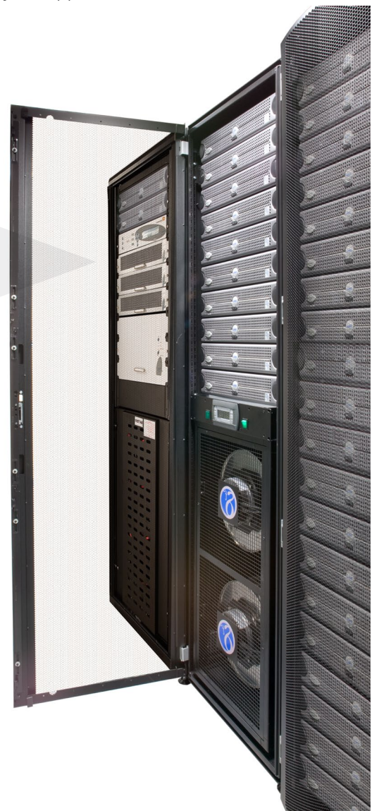
Installation view of a 24kW Datacube
